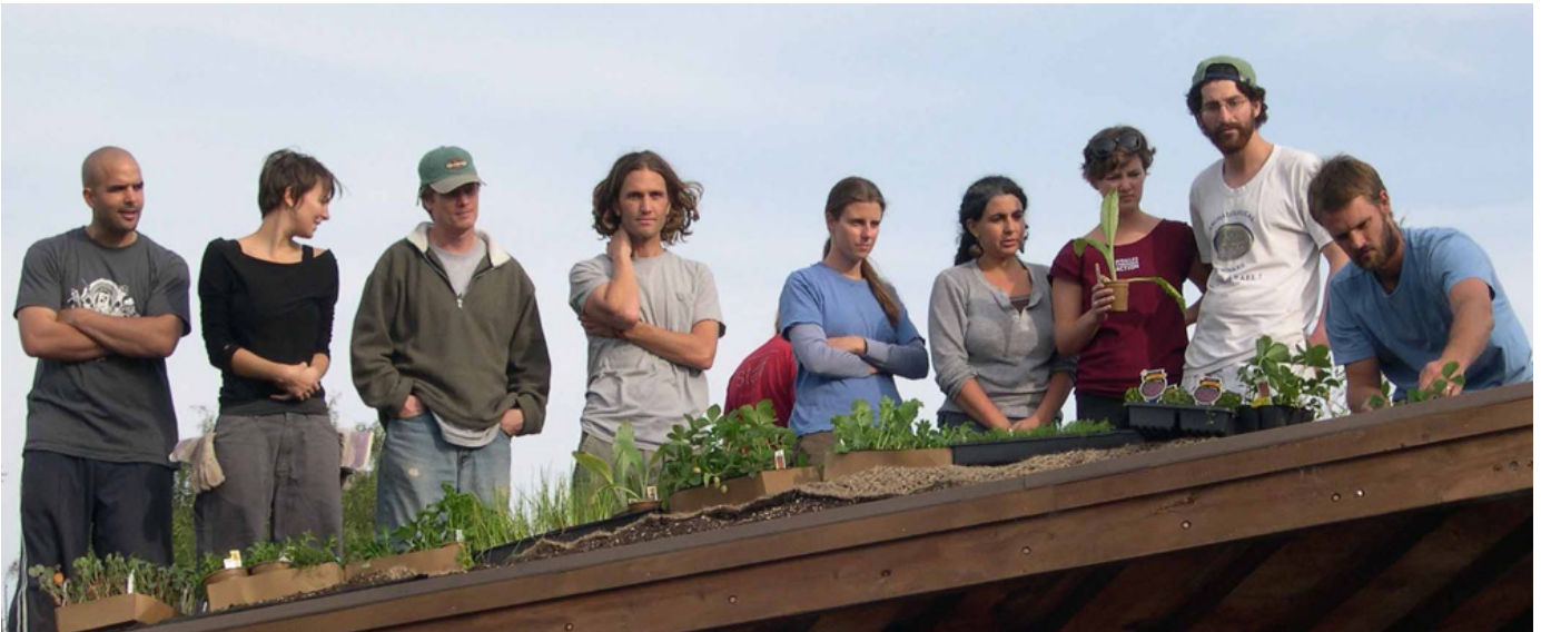
Volunteers install the living roof on the shed at the Eco House. Photo: Ingrid Severson.
