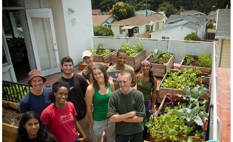
Building a school rooftop garden at E.C. Reems Academy in Oakland. Photo: David Hanks, www.davidhanks.org .
